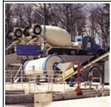
This RA-20 zero discharge plant with drive over surge hopper recycles all gray water and captured storm water.
